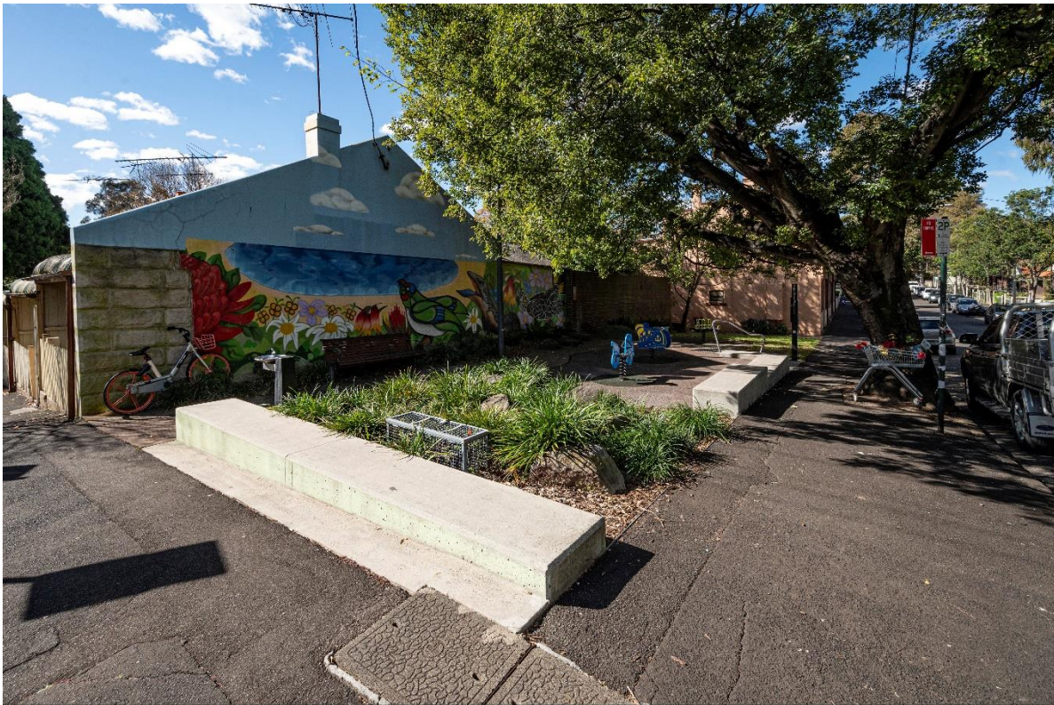
Looking east from Mitchell Street. Play equipment is at the end of its useful life and soft fall is worn and separating at edges. Planting areas are in reasonable condition. There is no paved access from Glebe Street. Low boundary walls are currently too low to be used comfortably as seating. There is one bench.
